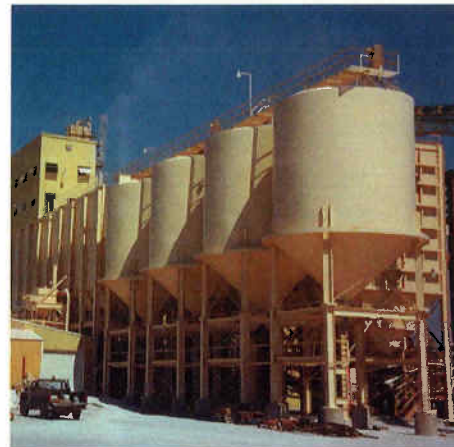
Above: 15' x 18' cone-bottom steel process hoppers – iron pellet storage
