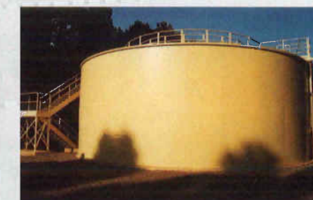
27' x 24', 100,000-gallon wastewater digesting vessel
