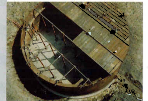
Above: 80' x 24', 900,000-gallon fuel storage tank
