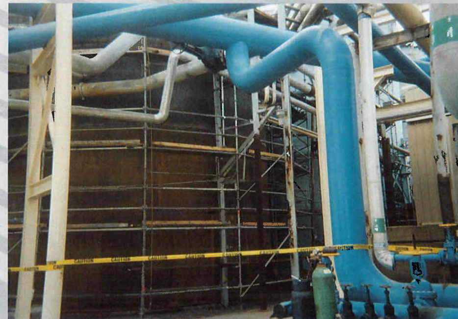
Liquor storage vessel – installed inside an operating pulp & paper facility
