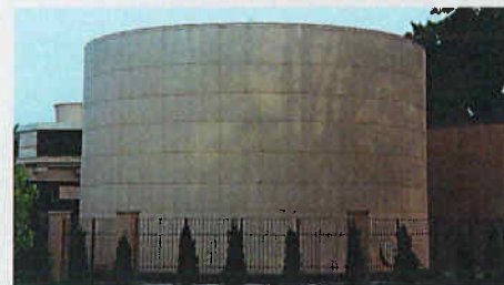
52' x 32', 500,000-gallon insulated chilled water storage tank – institutional power facility
